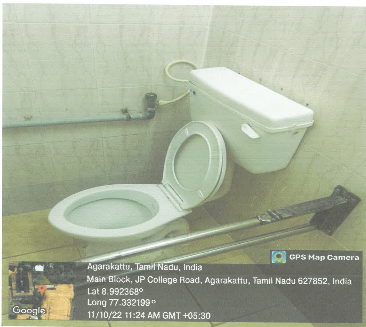
Disabled Friendly washrooms with handrails support
